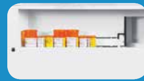
Open Control Center
